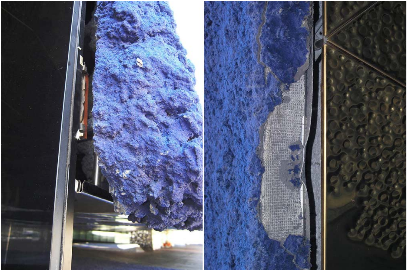
Figure 1. Details of the sprayed concrete Klein-Blue coloured façade of Forum 2004 in Barcelona by Herzog & de Meuron. Photo © Katia Gasparini
