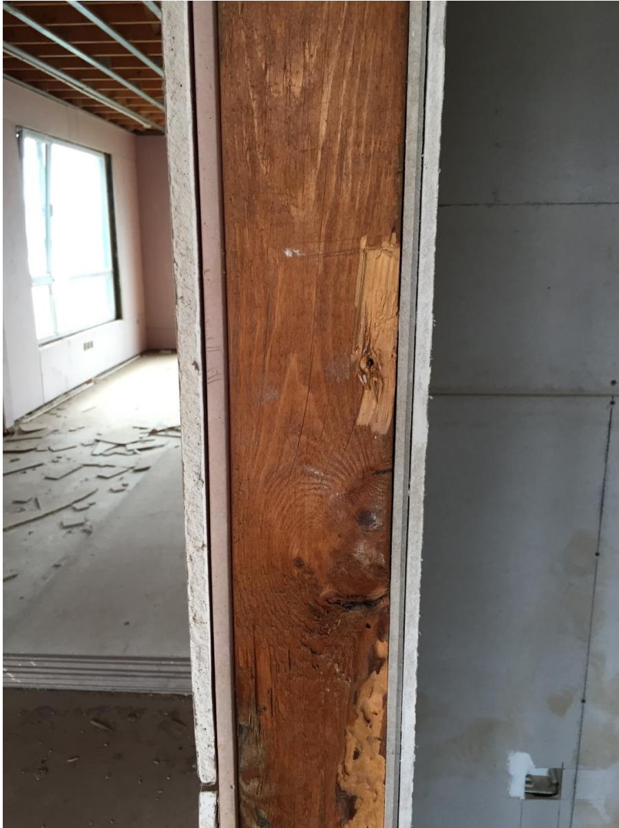
Image 6.1 The construction of The Aqua deviates from the local approach (Author's Photograph)
