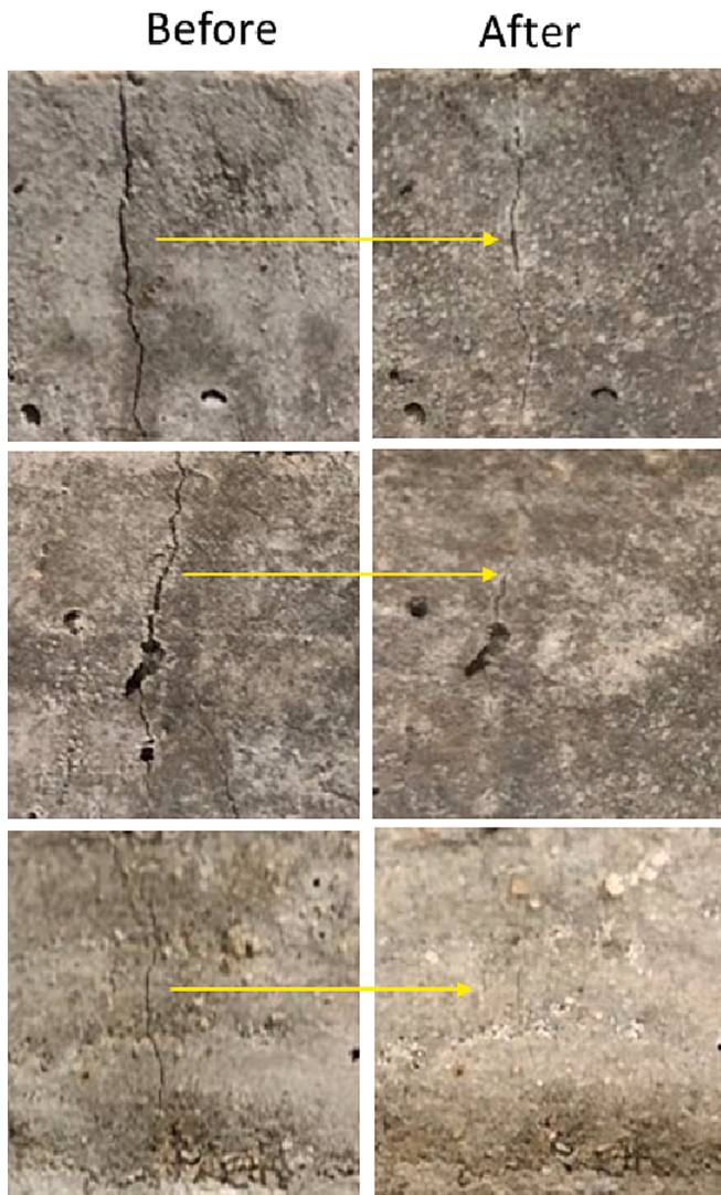
Fig 5. Observation of crack healing before and after incubation for bio-mortar specimens.
